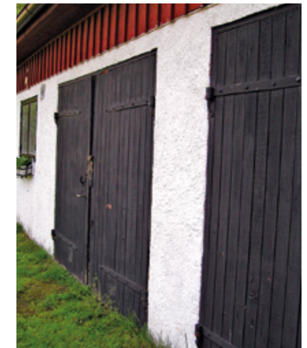
Garage Linseed Oil Emulsion Paint after 14 years
